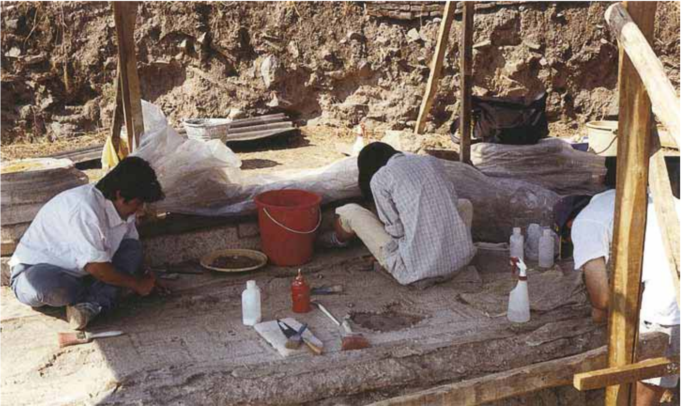
Figure 1: Cleaning and consolidation of mosaic floor in situ . Sardis, Turkey. Credit: Kent Severson
